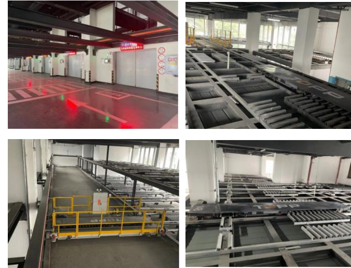
7、Government parking garage project in ChongQing, PPY-7, 7 floor, Number of Parking Lot 310
